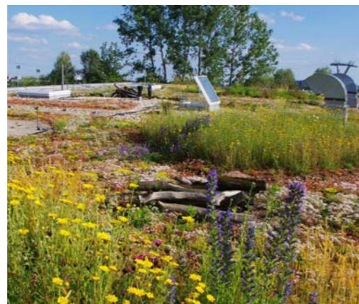
Low-intensity, low-weight options for exploiting extensive flat roof areas to create new types of habitat
